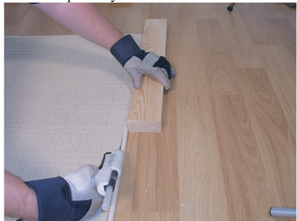
11) For large runs, try a piece of 2"x 2" to help attach large sections of the binding. Use a glue gun and pad to catch any glue that might drip from the end of the gun.
