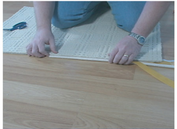
4) It is important to run the rope parallel to the carpet edge leaving sufficient gap between the carpet and the rope for the glue gun nozzle.
